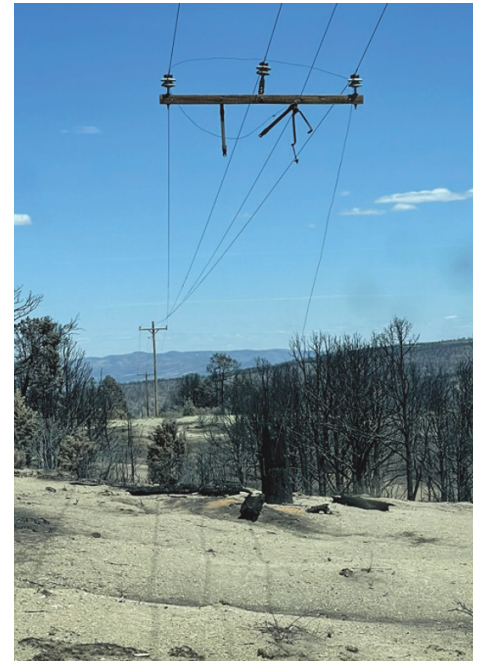
The fires caused more than $23 million in damages to WREA infrastructure.
